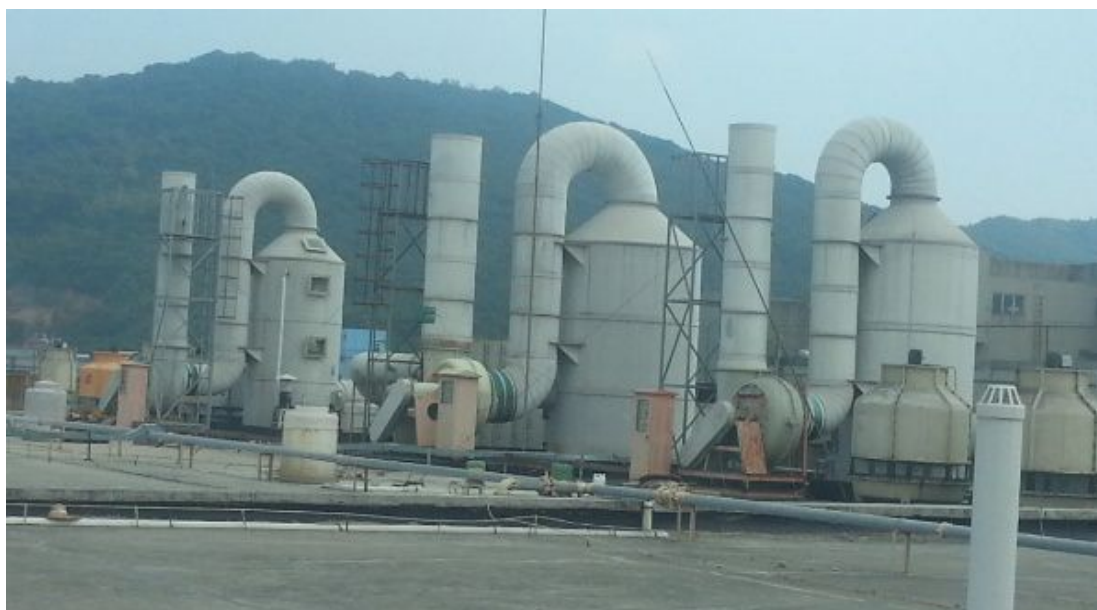
废气净化洗涤塔↑
